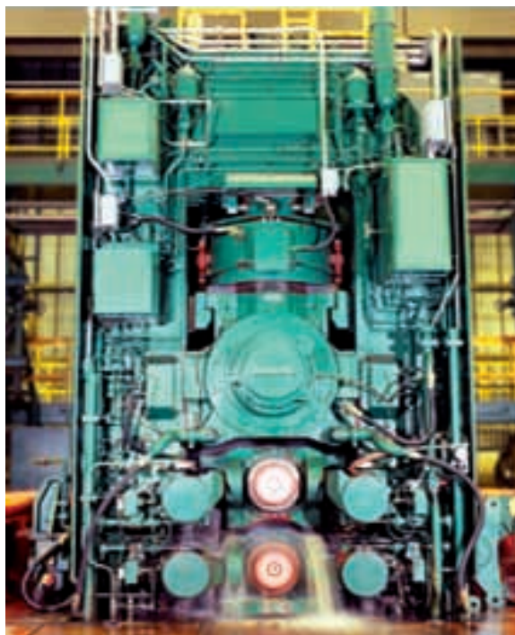
Morgoil bearings in a continuous hot-strip mill
