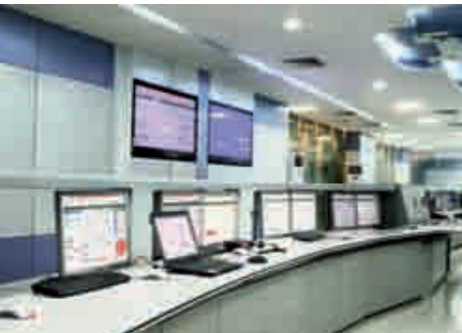
State-of-the-art automation system
