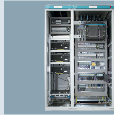
ALU TCS control cubicle
