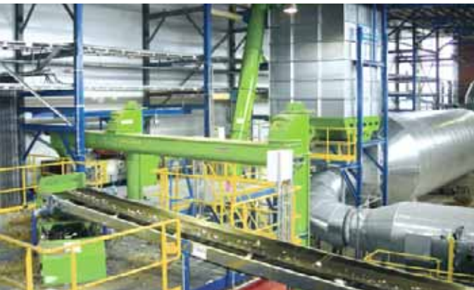
Reject To Fuel plant near Groningen in the Netherlands, with a capacity of 100,000 metric tonnes annually, for the production of high-calorific fuel from paper waste.
