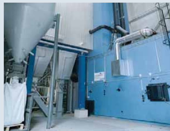
Combustion, burn-out and steam generation at the waste incineration plant in Hirschwang/Austria
