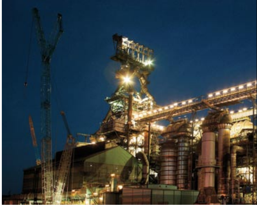
Blast furnace A, voestalpine Stahl, Linz, Austria
